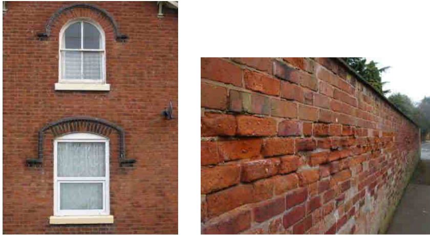
Fig. 14 Comparison and original and replacement upvc windows; decay of a brick boundary wall
