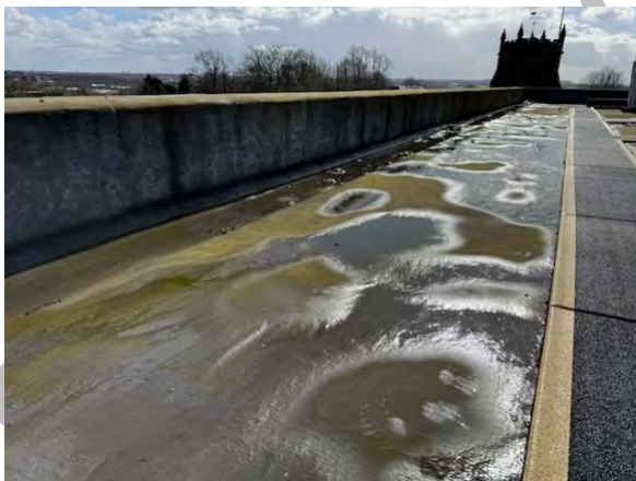
Fig 15 - View of blistering noted to the roof coverings. No edge protection is provided to the shallow parapet.
