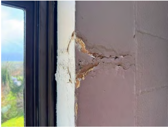
Fig 27 - View of penetrating damp around window apertures
