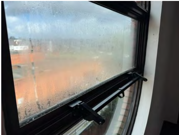
Fig 23 - View of interstitial condensation to second floor window.
