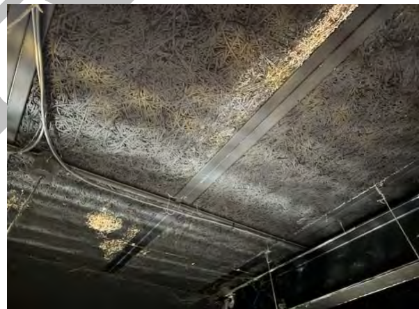
Fig 16 - View of the channel reinforced woodwool slab roof deck and evidence of previous rainwater ingress.
