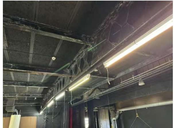
Fig 28 - The paint finish to the steelwork is in poor condition.
