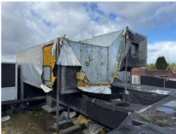
Fig 17 - View of roof mounted plant and poor condition of insulation.
