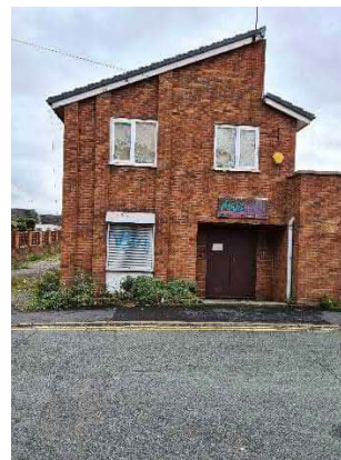
Photograph 8: Derelict building in poor repair along Price Street
